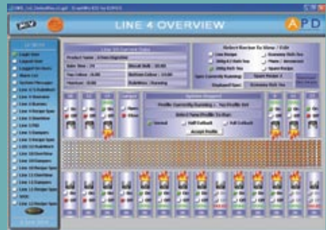
Burner Control Screen
