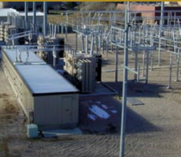
A Fort Collins Utilities Monitored Substation
