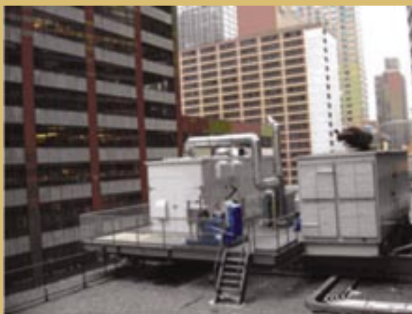
A DFC300 installation in downtown Manhattan
