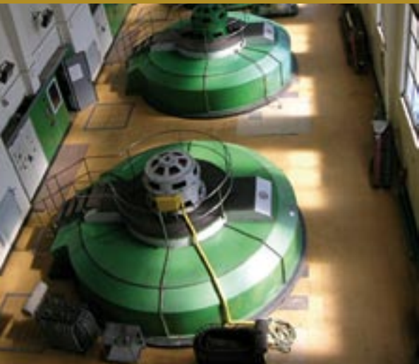
Hydro Turbines at an E.ON Hydro Power Station
