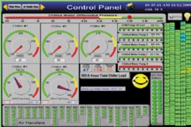
Longmont United's self-built control panel
